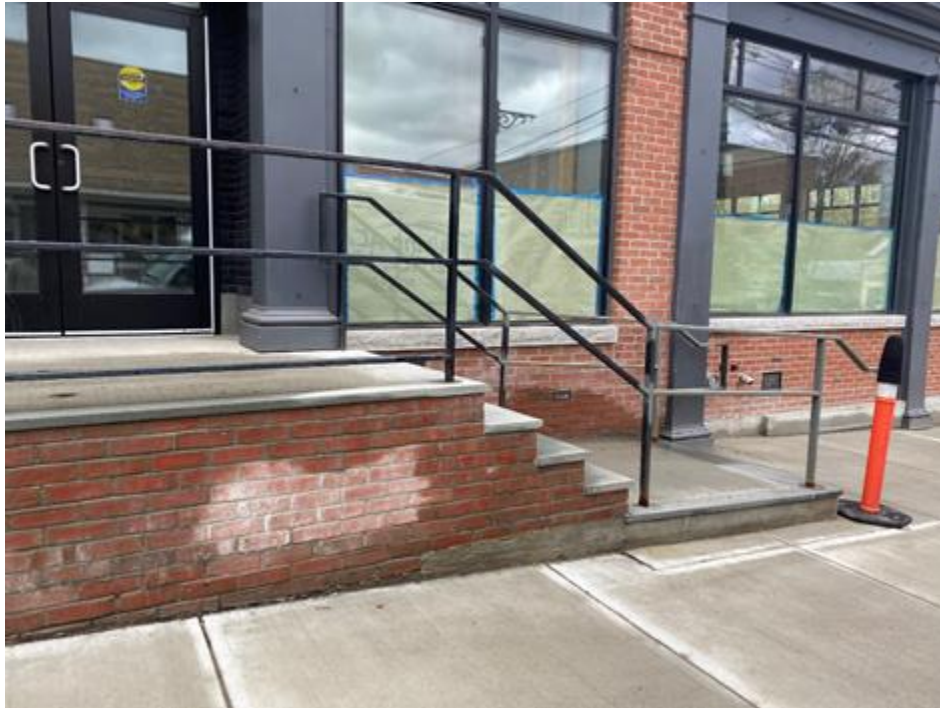
The Vault building (former TD Bank), 14 South Main Street, front entry stairs.
