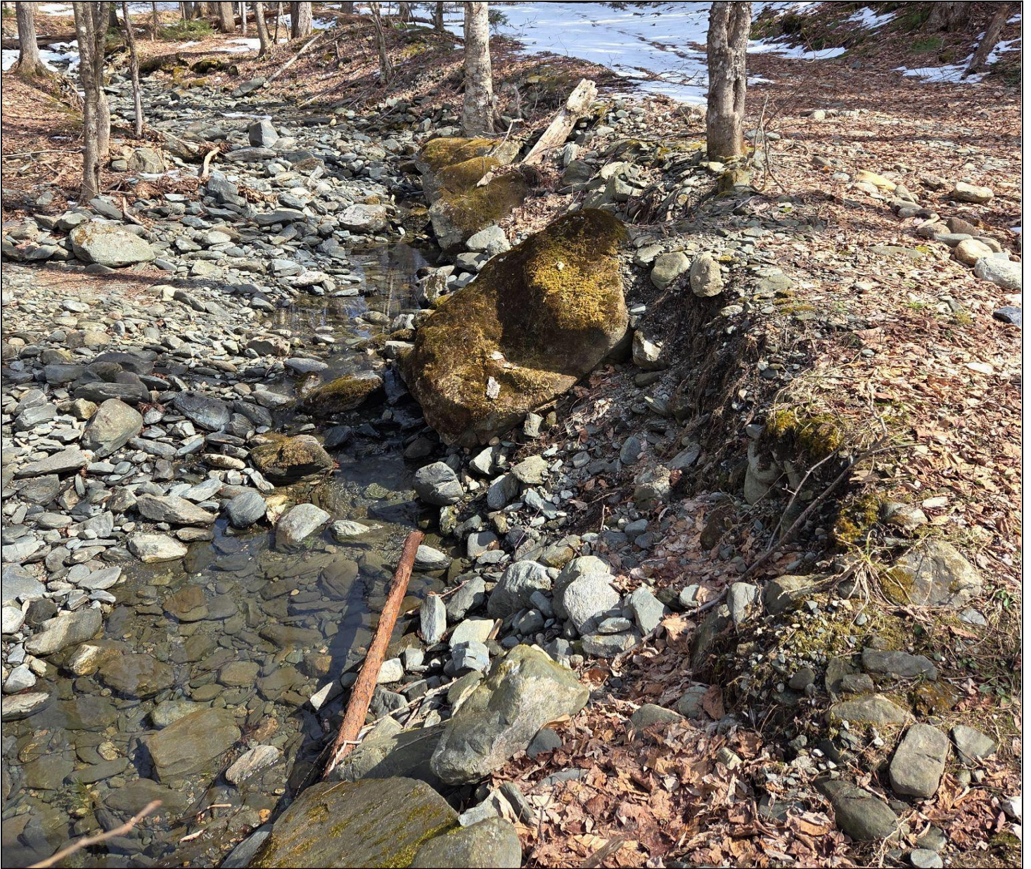
Figure 43: Streambank erosion and road-edge cave-in along Tyler Brook just north of Waterworks Road (sandier soil section of parcel).
