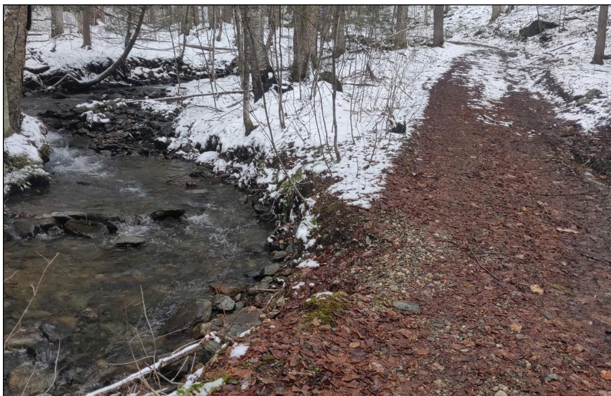
Figure 41: An access road eroding into Merriam Brook, near the parking lot (below the dam).
