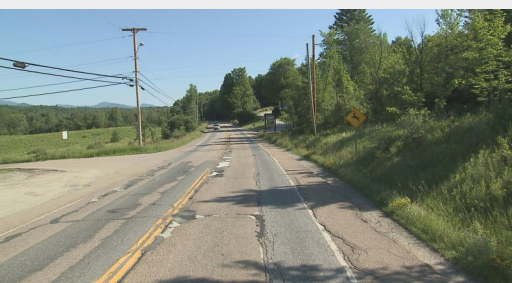
Deteriorating roadway pavement
