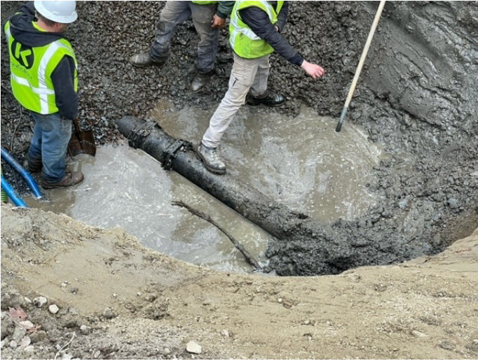
Water from the brook infiltrating the hole
