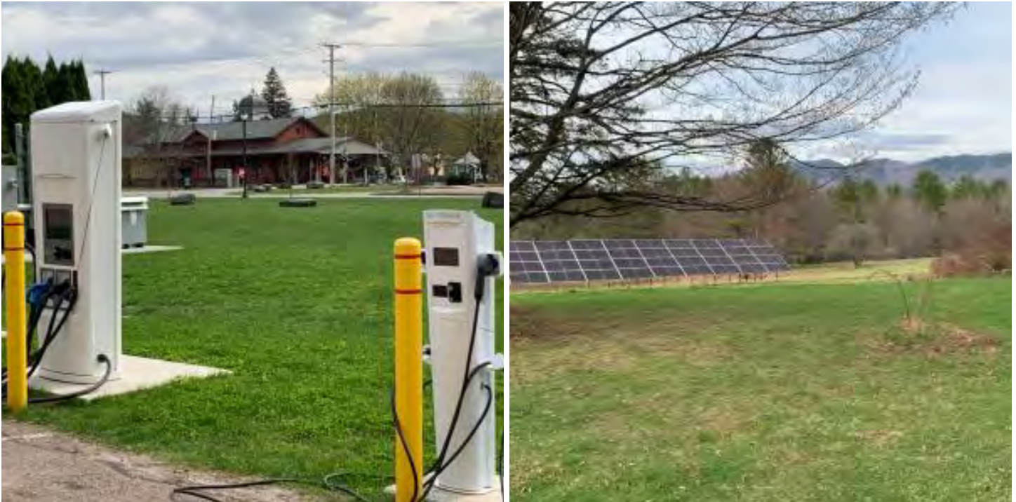
L: EV charging in Waterbury. R: A solar array in Waterbury.
