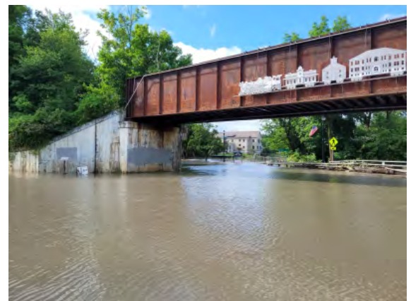
Flooding in July 2024 submerged parts of the Roundabout at the entrance of Waterbury. Photo: Emma Malinak / VT Digger
